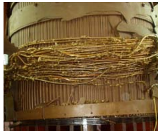
Collapsed tap winding
